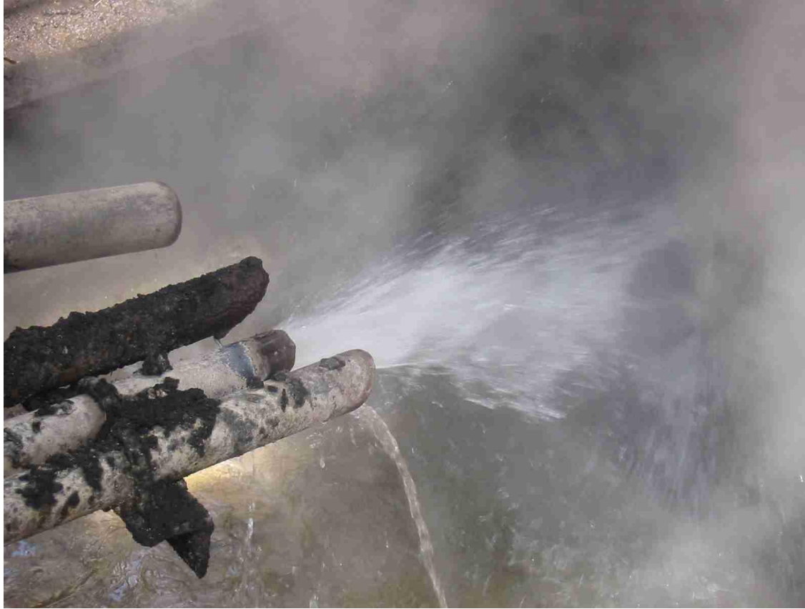
Hot water flowing out of a pipe
