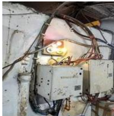
After: Electrical panel with LED lights
