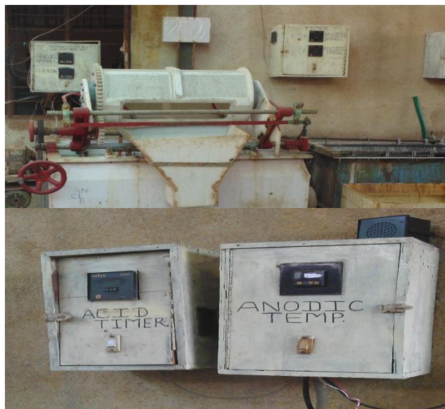
After: Installation of a timer and buzzer at all process tanks, including degreasing and anodic cleaning tanks.
