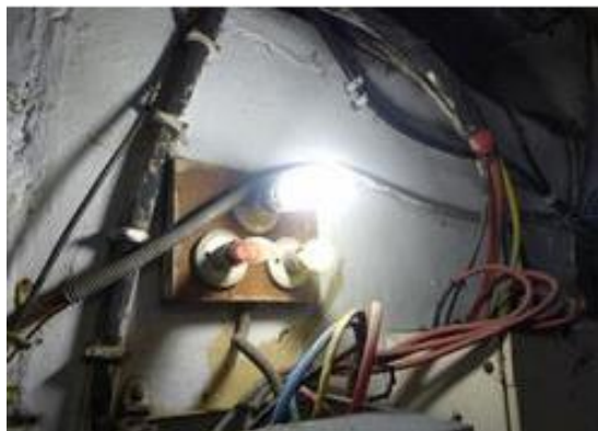
Before: Electrical panel with one CFL and two incandescent light bulbs
